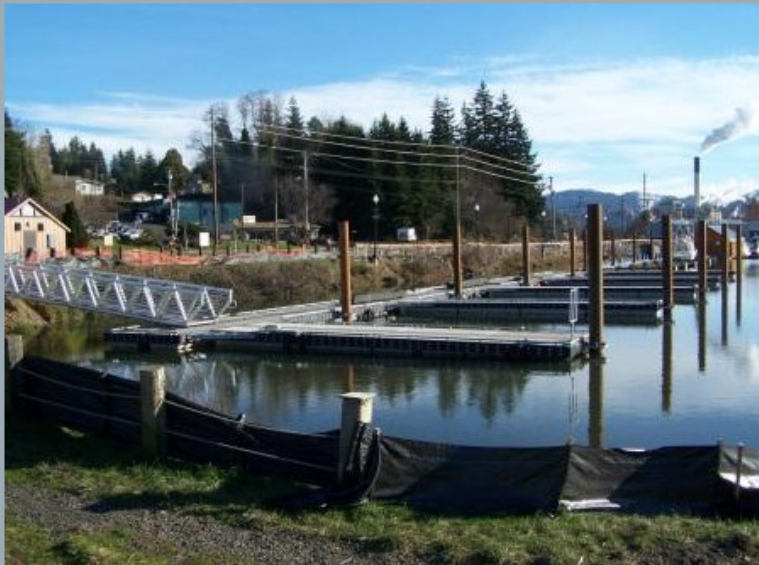
Current view of the Transient Dock, looking South from the Park Pavilion that is under construction.
