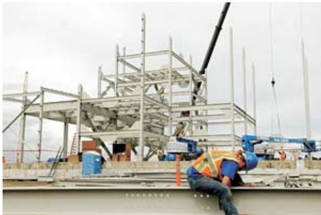
World Photo by Benjamin Brayfield A construction worker prepares beams Sept. 15 before they are set in place as part of the Oregon Resources Corporation processing plant.
